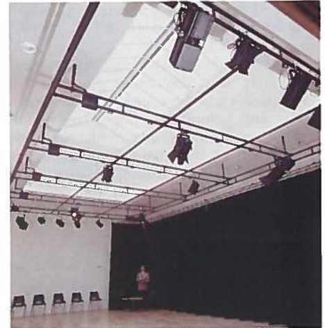
Rehearsal Studio 2 showing lighting grid and perimeter drapes.
